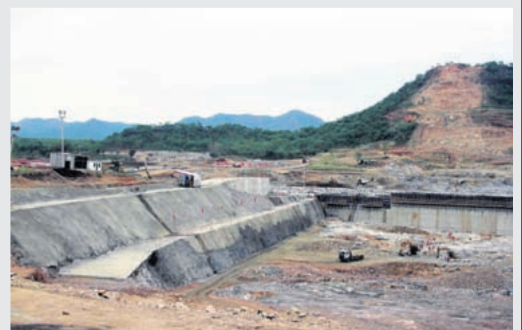
In this June 28, 2013 file photo, construction work takes place, at the site of the Grand Ethiopian Renaissance Dam near As-sosa, Ethiopia.
